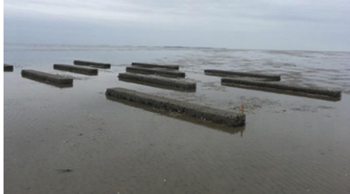
Figure 28. Picture of placement of biodegradable BESE elements on mudflats in the Wadden sea (Nitsch et al., 2021).
